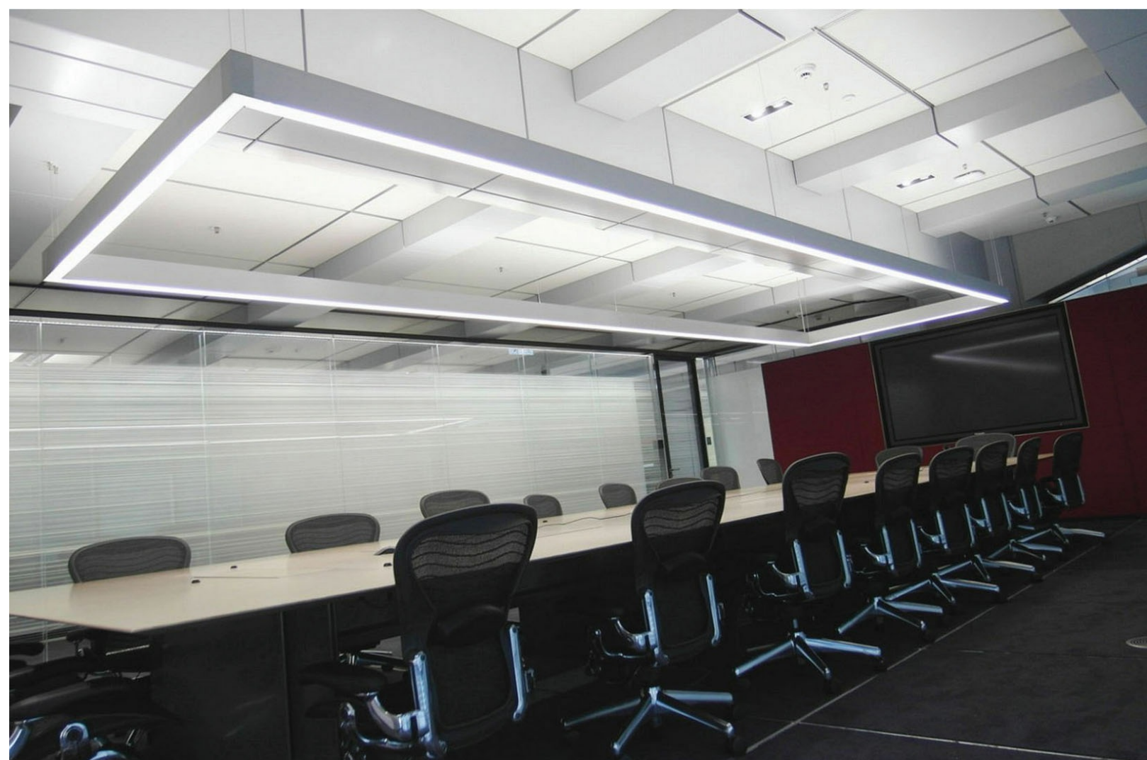
Figure 4.36 HSBC video conference and meeting room. Rectangular pendant supplies the vertical light level needed. Illuminated wall divider and spotlights provide back lighting.
